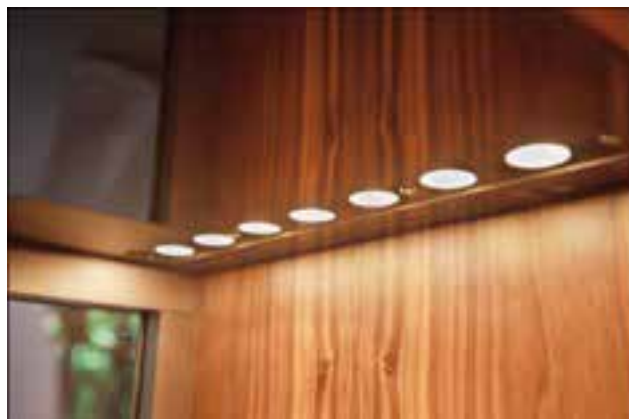
Barra Luminosa LED 7W - instalada
